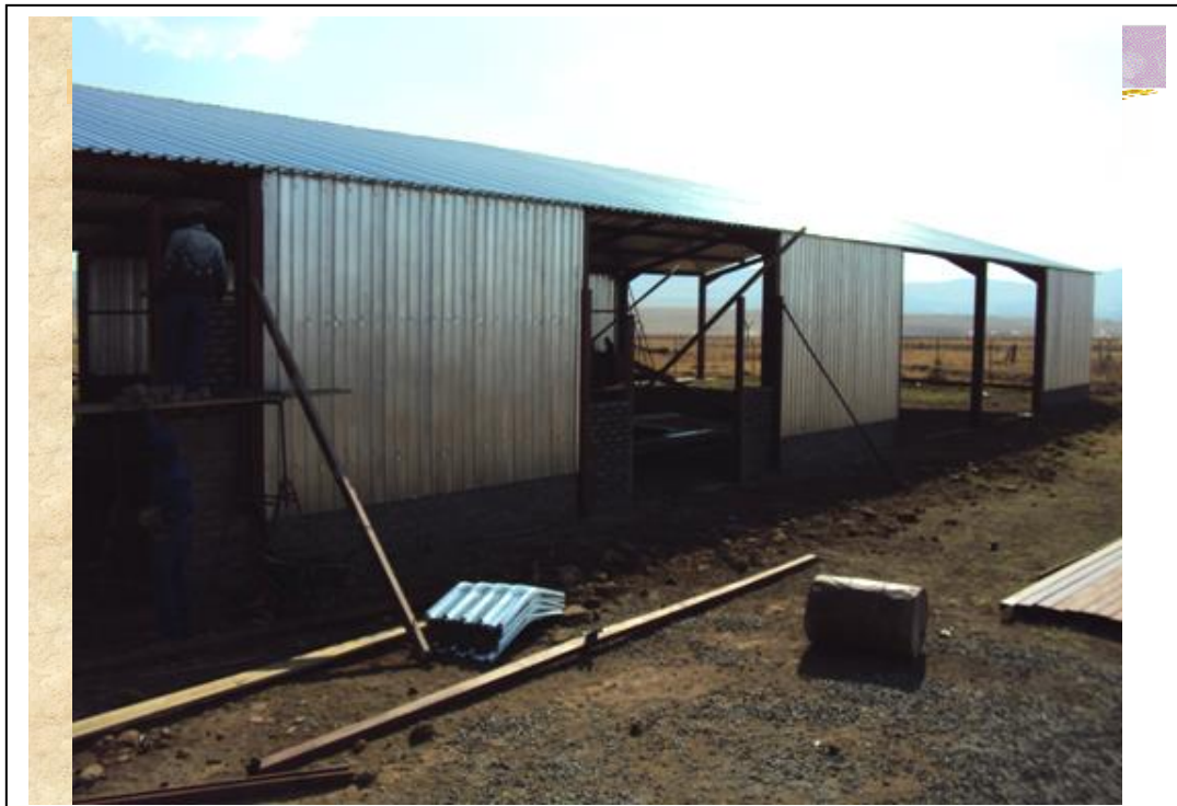
Photo: Construction of the Sisonke Support Centre and Cooperative in progress. The maize mill will be installed to the entrance on the left side.
